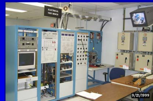
Electrical Sys Test Bench
