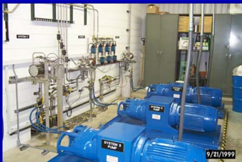
Hydraulic Pump Room
