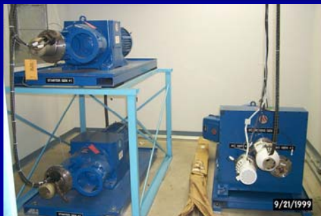
Electrical Generator Room
